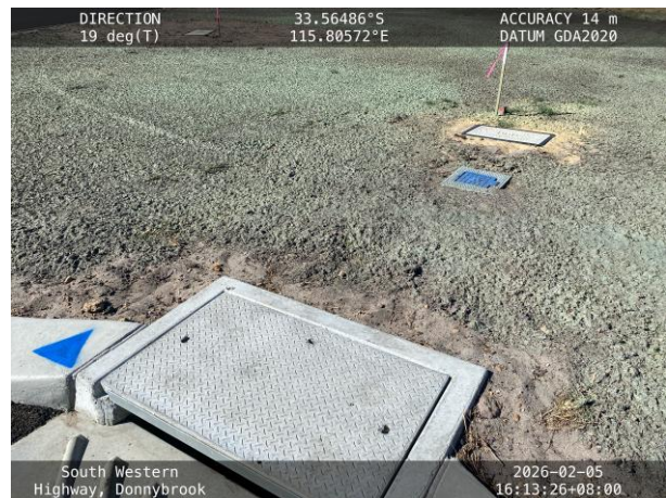
Photo 4 - Fire Hydrant with verge marking
